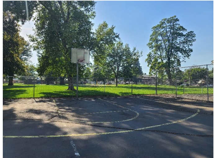
Basketball courts with cracked surface; dilapidated fencing.
